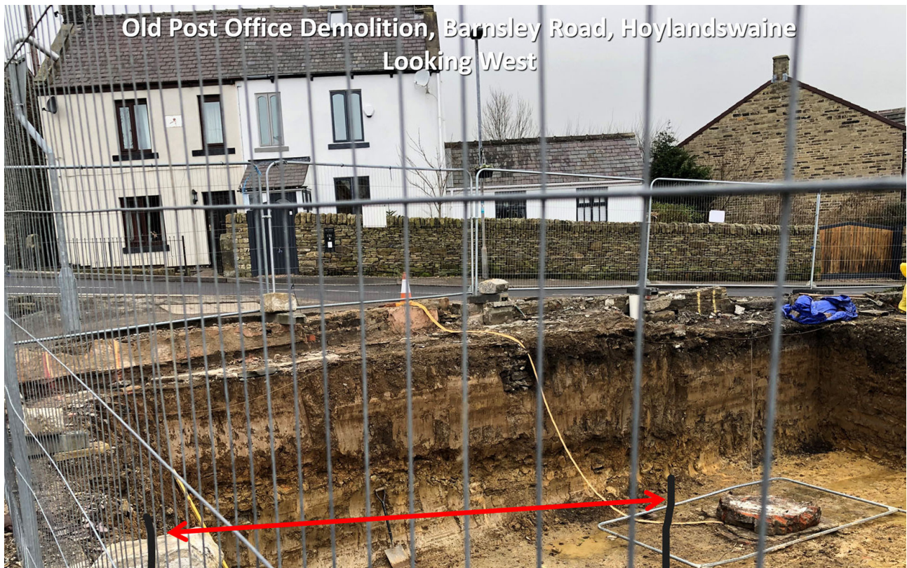
Fig 3: The excavated cellars of the Old Post Office. The red arrow marks the 7 metre width of the surviving Roman road in the side of the excavation. Image by Philip Jones
