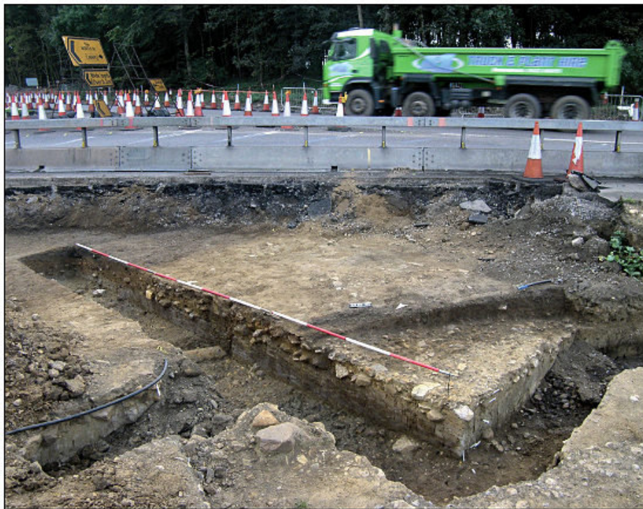
Roman road 6 sectioned heading north east from the modern Scotch Corner roundabout. View looking south east. Work underway alongside live traffic. Copyright Northern Archaeological Associates
