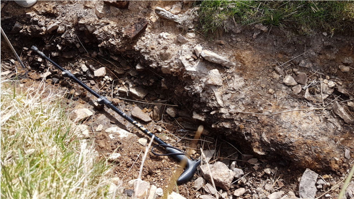
Fig. 3, Drainage channel cut across the road showing elements of its construction, stick set at 1metre length
